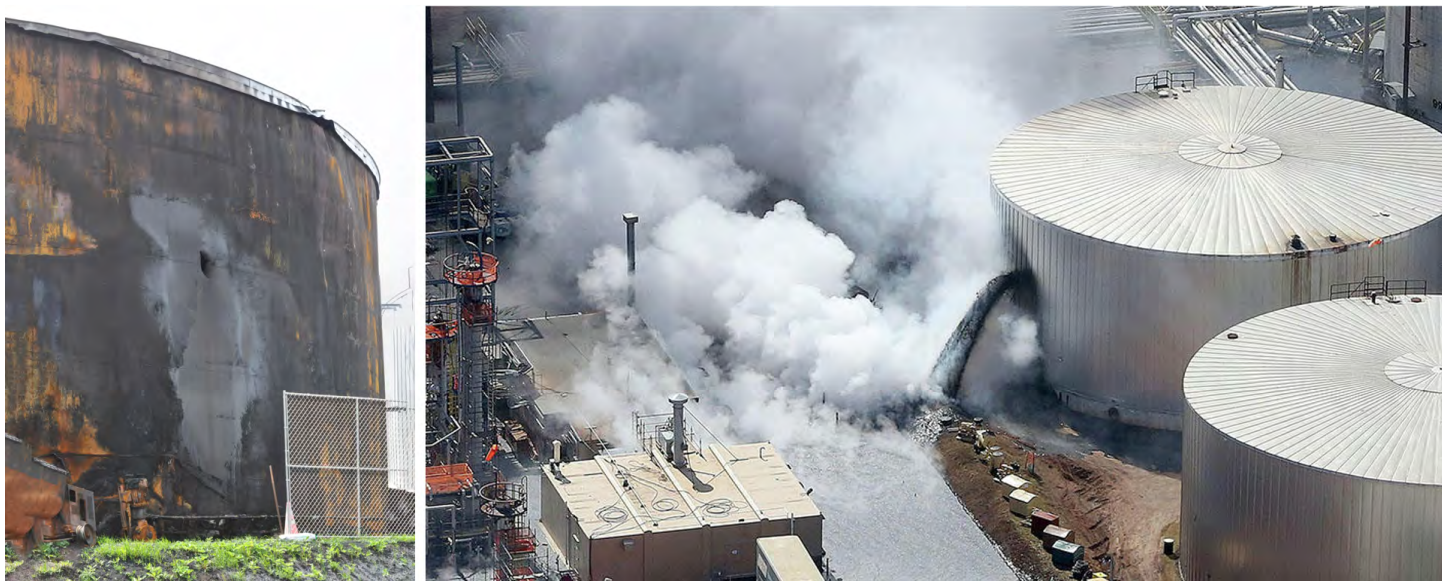
Figure 4. Post-incident photographs of the leaking Asphalt Storage Tank. Debris from the explosion punctured the side wall of the tank creating a large asphalt leak outside of the secondary containment area. Credit: CSB (left) Duluth News Tribune (right).
